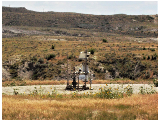
Fig. 4. Wellhead in the Salt Creek oilfield of Wyoming, USA, with infrastructure for injection of CO 2 to carry out Enhanced Oil Recovery operations. Source: Photographed by Dan Soeder in 2019.
